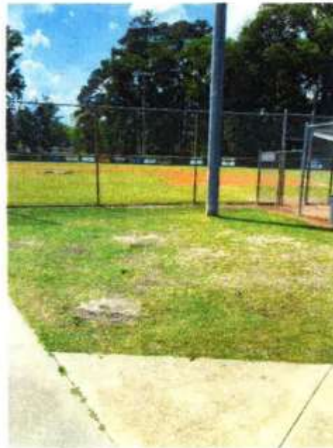
Dugout improvements. Concrete ADA Sidewalk Access to Dugout with new brick Compatible dugouts to facilitate ADA access
